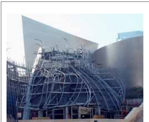
Disney Building, Los Angeles under construction revealing a smooth skin over a chaotic structure 2002. Frank O Gehry and Partners
